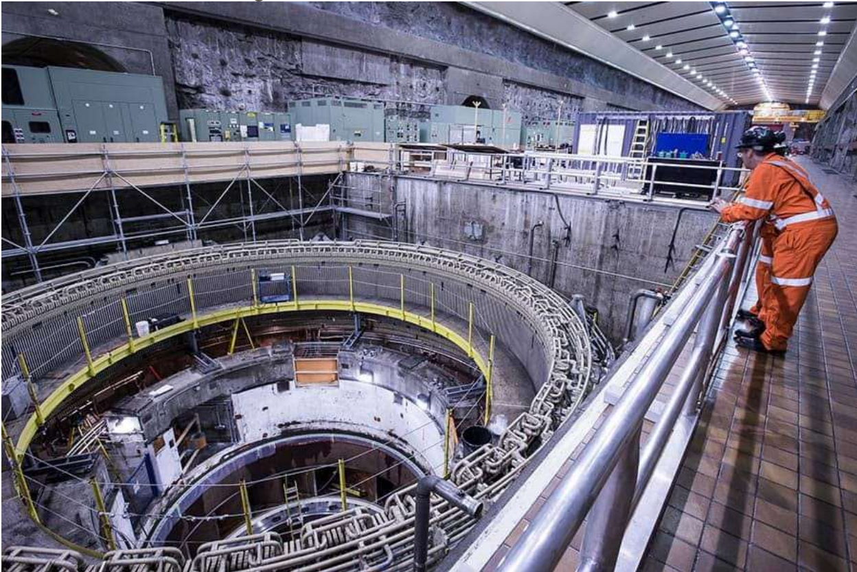
Interior of a hydroplant turbine vault (La Grande/Robert-Bourassa)
